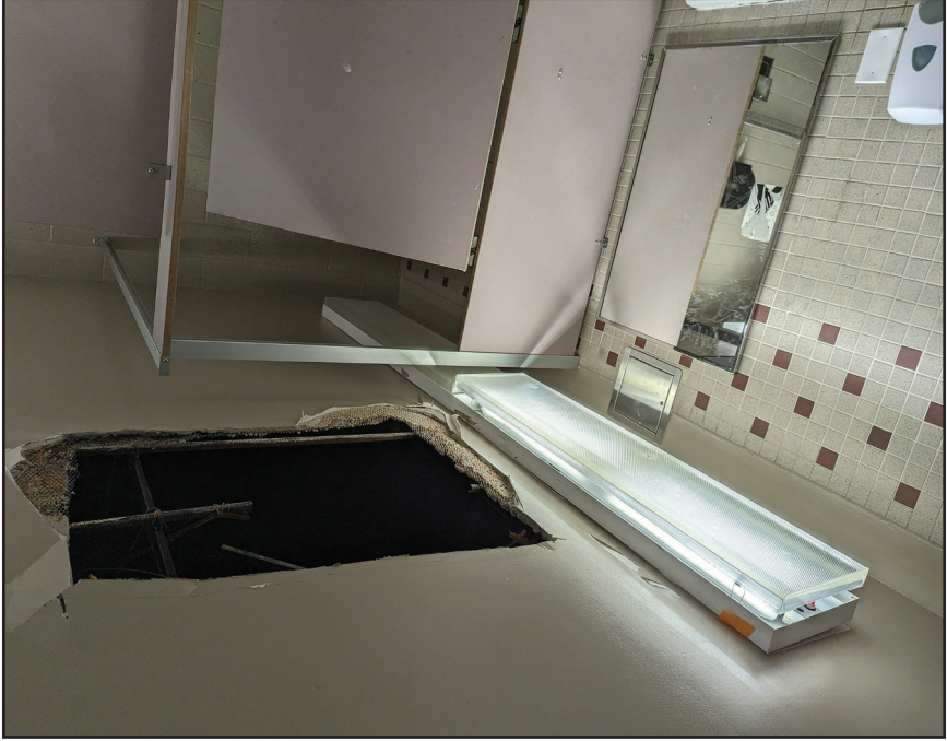
Bathrooms in the 50-year-old C Building were closed earlier this semester for repairs. / Zandy Garrido / el Don
